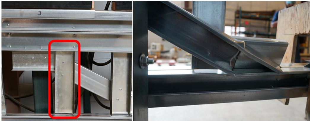
Figure 6: a) Second Reinforcement, b) Web Failure After Second Reinforcement
