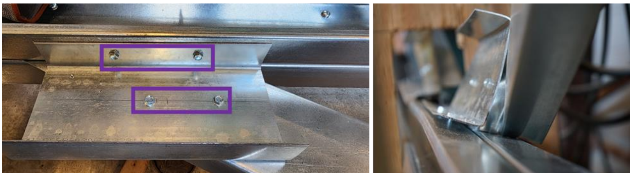
Figure 5: a) Clip Angle Type of Reinforcement, b) Failure of the Reinforcing Member
