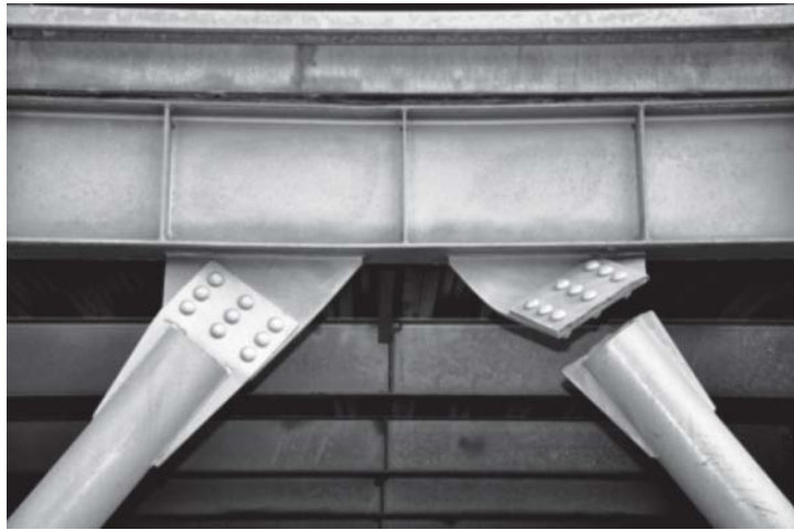
Figure 4: Damage in a steel brace due to seismic forces
